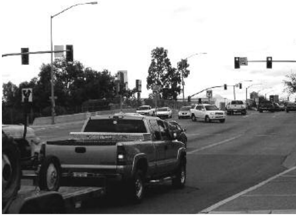
The Sixth Avenue exit off I-10 will soon be jammed with traffic when all exits between 29th Street and Prince Road are closed for three years for the I-10 widening project.
